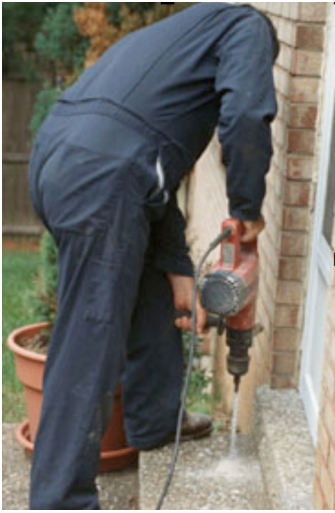
PMP drilling the steps so that he can inject liquid termiticide against the foundation wall.
